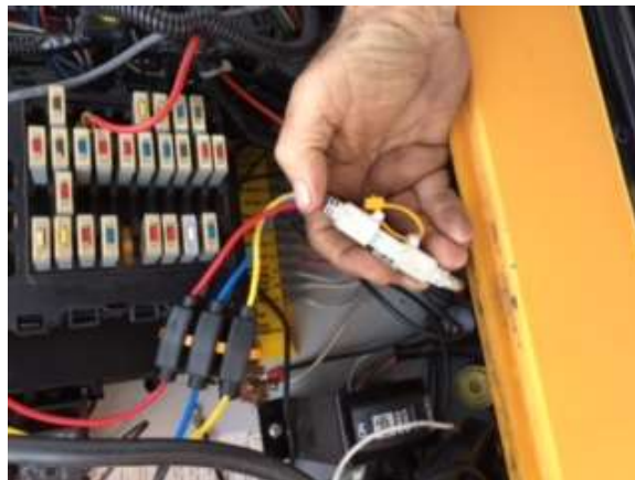
Corrective Action: Reconnected Wiring with a Zip-Tie
